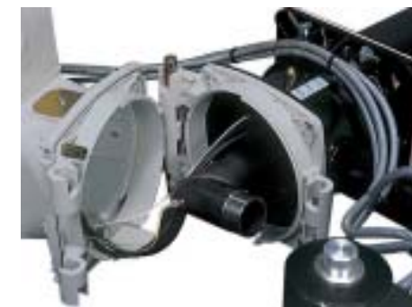
Combustion head inspection
